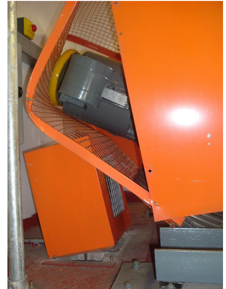
The entire drive unit had collapsed
