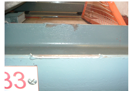
The welds had not penetrated
